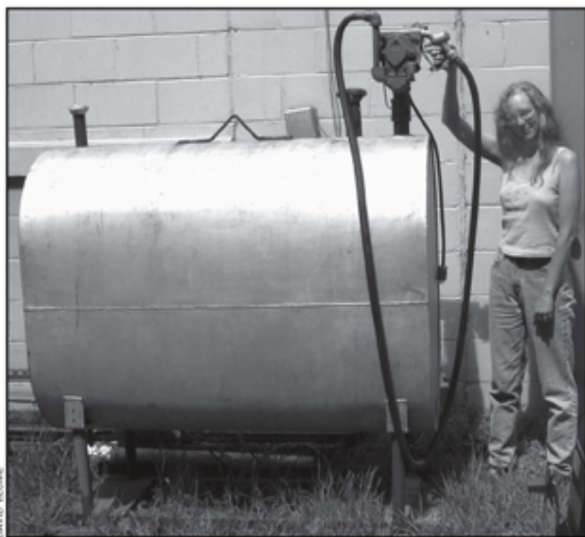
Fig. 29-9 Fuel oil tank alcohol dispenser. These mass-produced 275 gallon oval fuel oil tanks are rated for flammable liquids. As you can see here, they make dandy private filling stations. Get a permit for it using fuel oil and add your electric pump and vent later, after approval. You can use the same tank to fuel your cogenerator.
